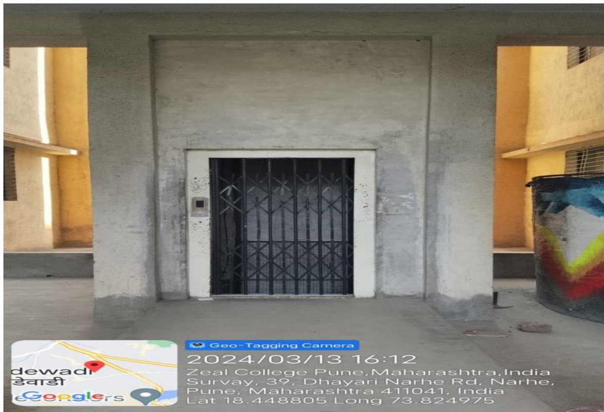
Image-7.1.7. (1-c) Lift made available for ease of access at entry point ZIMCA
