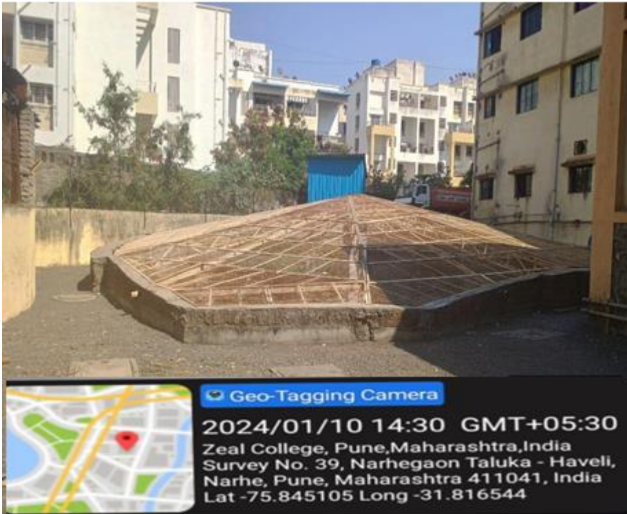
(Open well for general water use arrangement in the Campus)
