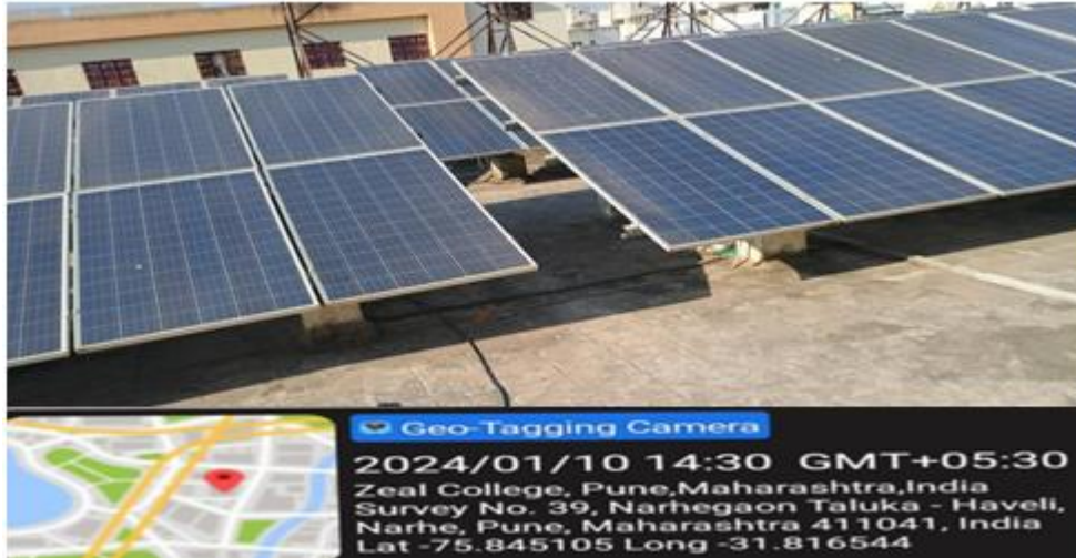
(120 KW roof top net metering Solar PV System in the Campus.)
