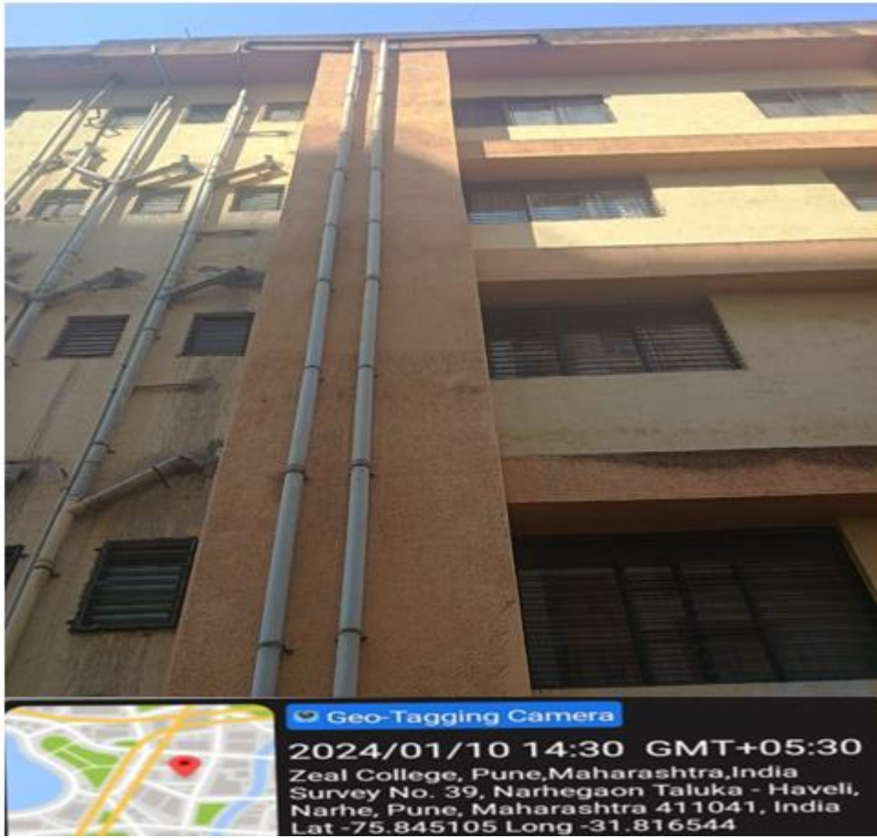
(Rainwater harvesting arrangement the in the college building)
