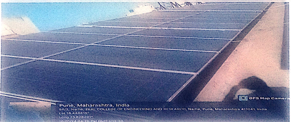
Solar panels at rooftop
