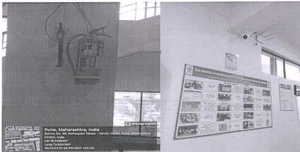
Safety Measures : Fire Extinguisher and CCTV
