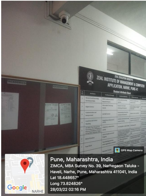
Image-7.1.1.3-CCTV at ZIMCA Corridor
