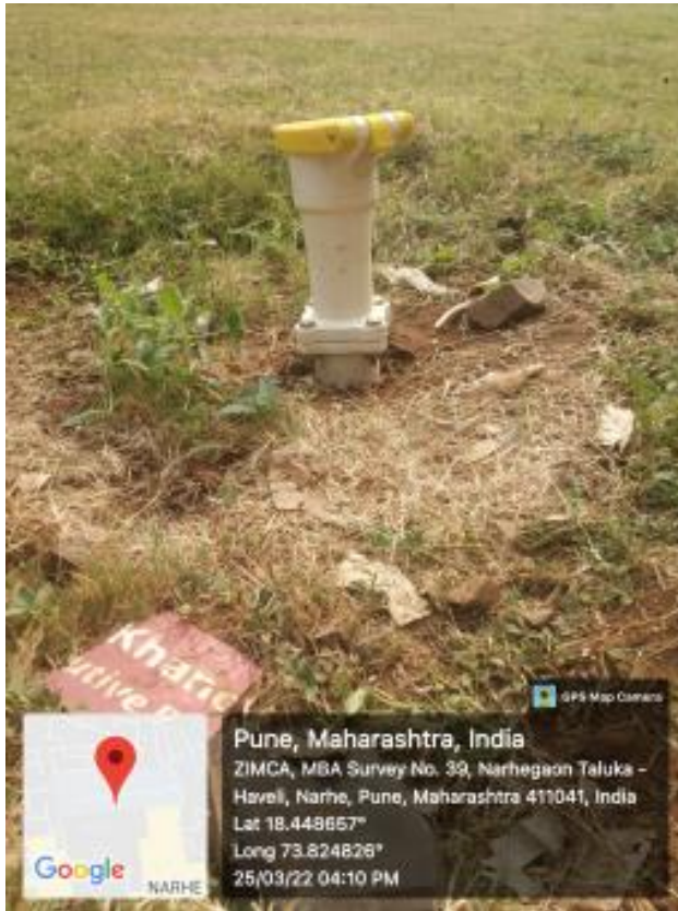
Image-7.1.1.8-Sprinkler System at ZES Campus
