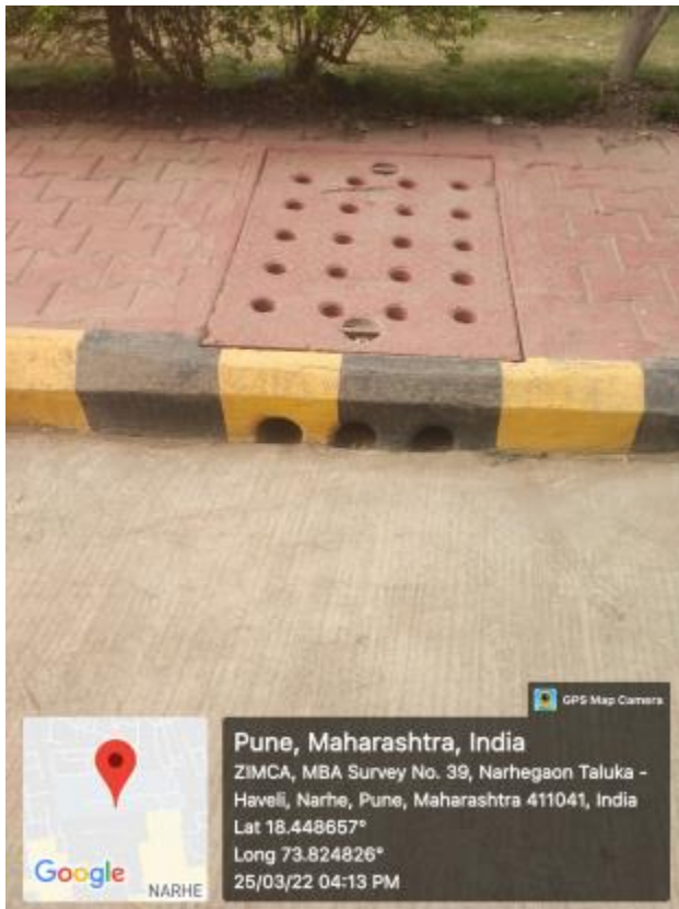
Image-7.1.5.5- Underground Drainage System at ZES Campus
