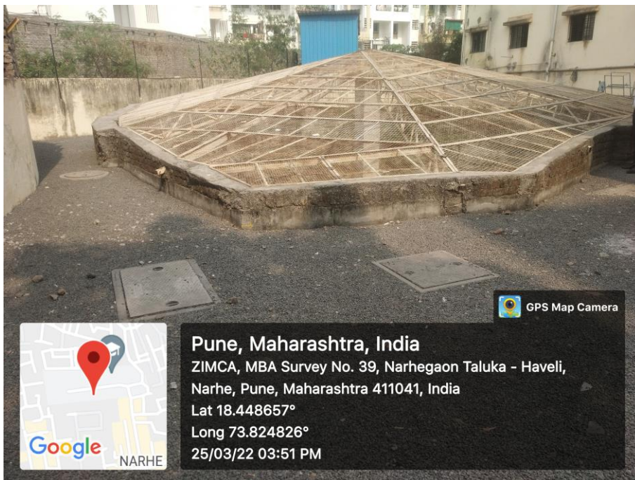
Image-7.1.4.2(c)-Open Well Recharge System @ ZES Campus
