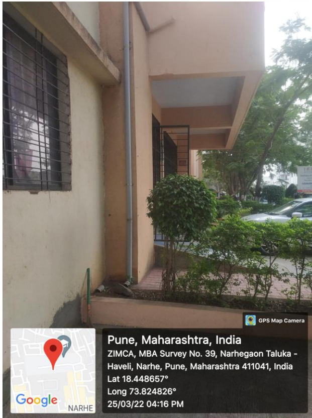
Image-7.1.4.1-Rain Water Harvesting System
