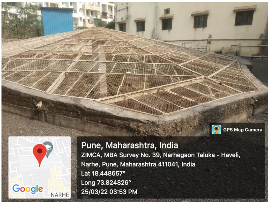
Image-7.1.4.2(a)-Open Well Recharge System @ ZES Campus
