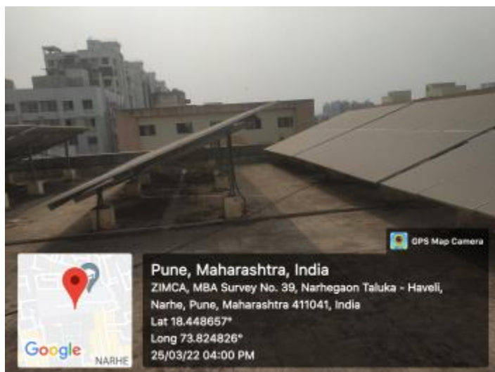
Image-7.2.1.1-Solar Panel at Roof top
