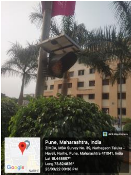
Image-7.2.1.2-Solar Panel at Signaling System
